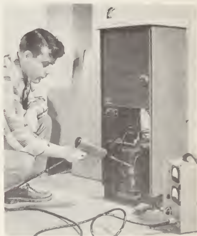
20-16. An electronic leak detector being used to check a self-contained water cooler. (General Electric Co.)
